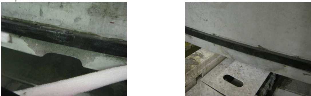
Figure 6. a) Concrete cover damage detected before installation b) Segment after repair
