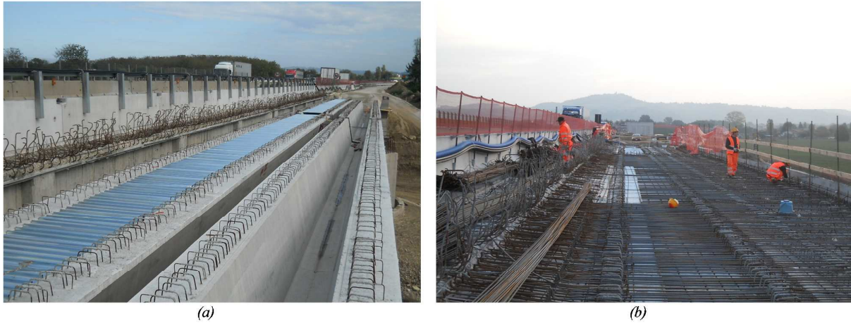
Fig. 4: Widening intervention of Foglia Bridge. (a) Prestressed concrete V-shaped girders. (b) Steel reinforcement of new deck slab.
